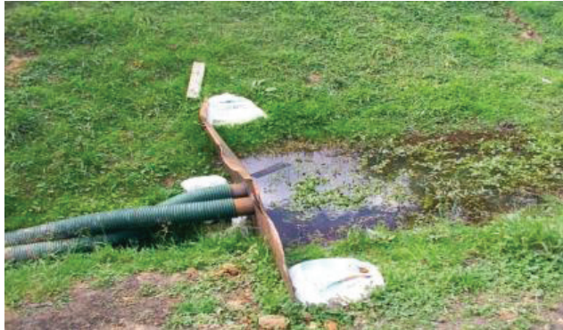
Figure 4 Example of dam and pumping diversion (New Zealand Transport Authority, 2014. Erosion and Sediment Control Guidelines for State Highway Infrastructure)
